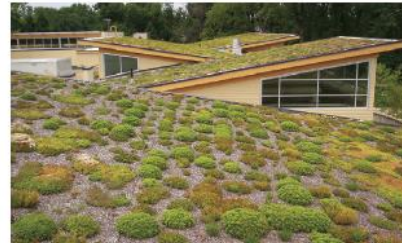
Green Roofs A vegetated roof, planted over a waterproofing membrane, which can help reduce stormwater runoff, lower cooling costs, and provide habitat for wildlife. Photo by Arlington County VA on Flickr/CC
